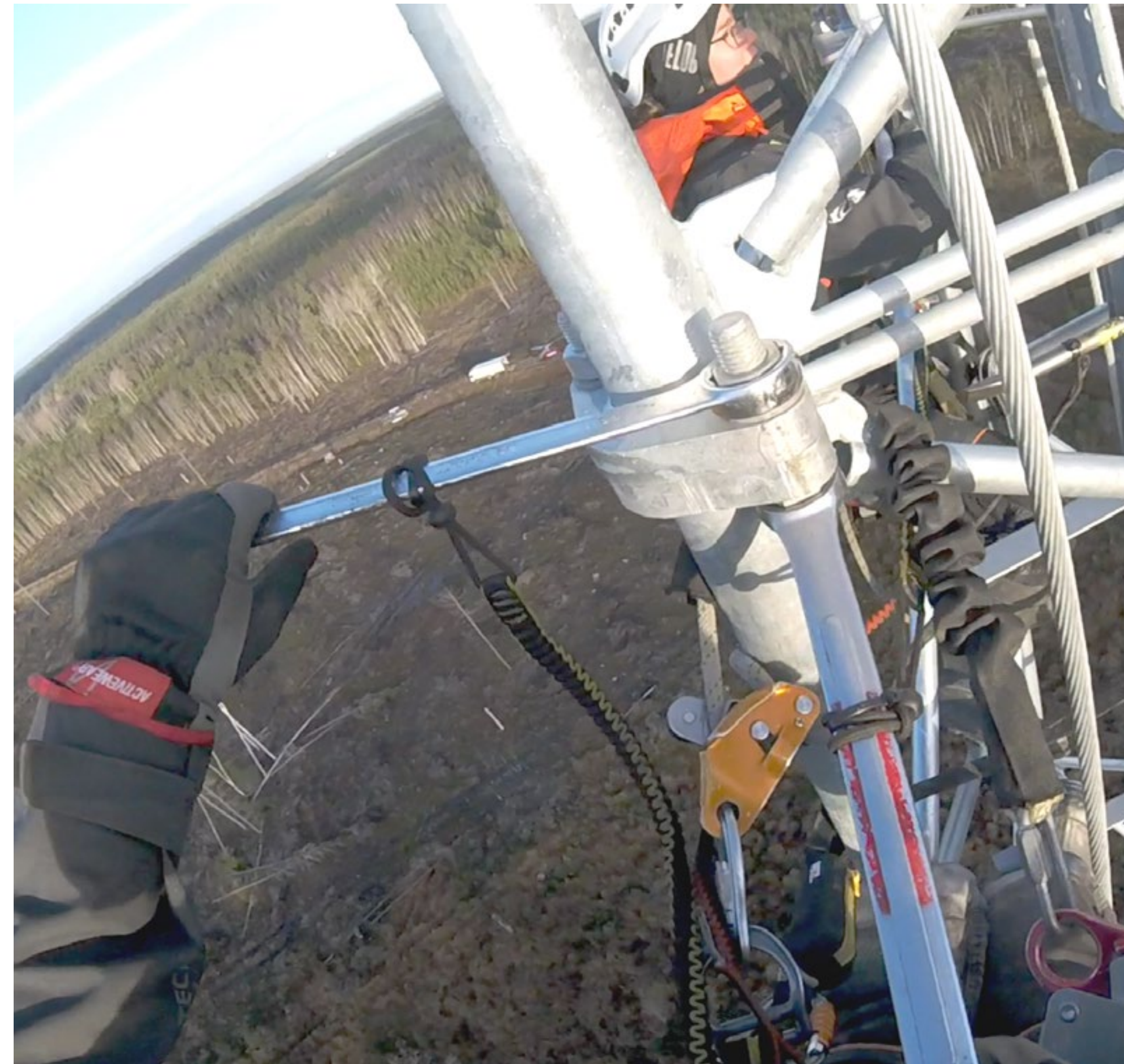
A mess of safety lines, tool tethers, carabiners and rappelling gear restrict freedom of movement. The highlighted wrench is borrowed from someone else while still tethered to that person.
